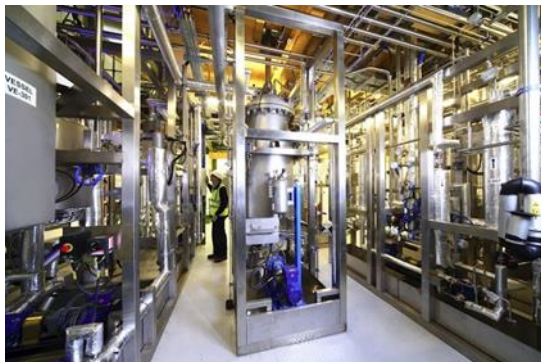
Figure 2: Optipure manufacturing facility
